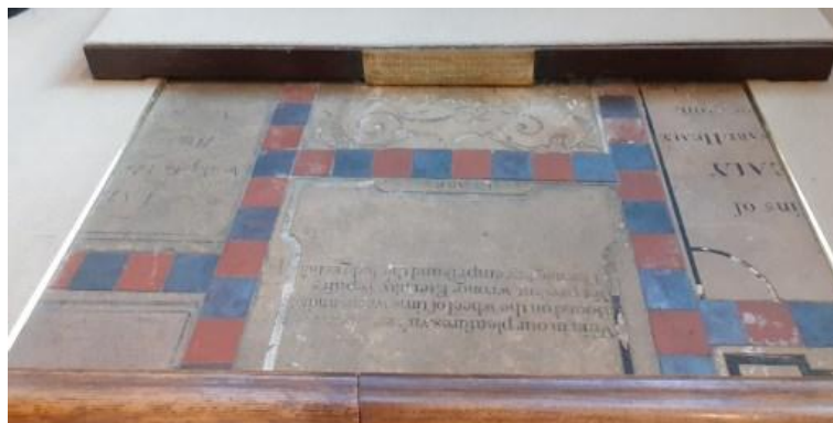
Figure 2 Detailed view of the slabs in front of the Lady Chapel altar
